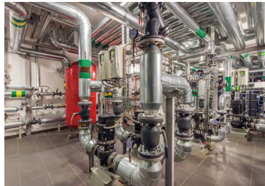
Municipal heating system
